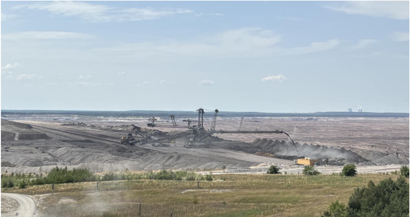
Figure 13 At the Nochten II opencast mine, soil is being spread over the mining wasteland for recultivation.
